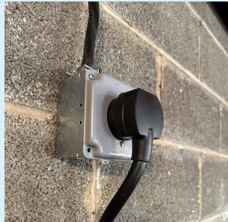
Example of a receptacle
