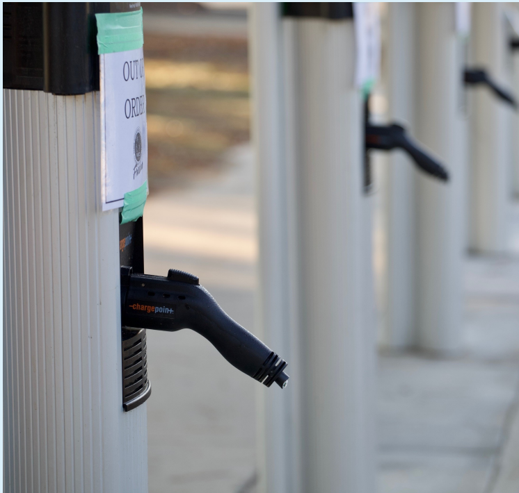
Example of cord vandalism in Fresno, CA (88 of 88 public chargers vandalized, $245k spent in remediation) 1
