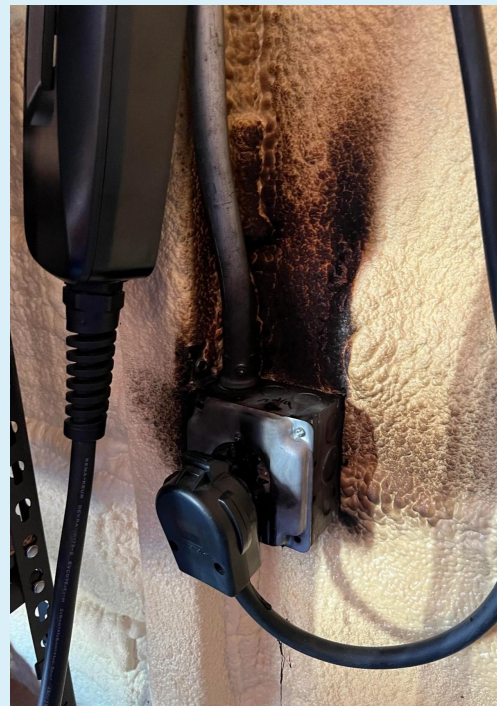
Example of a NEMA Receptacle experiencing “thermal issues”
